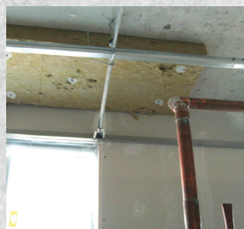
Above acoustical ceilings
